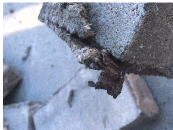
Figure 5 – Deteriorated steel wall tie
