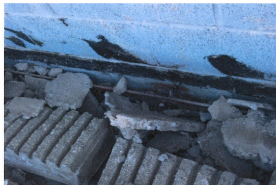
Figure 4 – The steel angle separated from the wall
