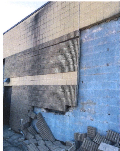
Figure 2 - Wall area likely to fall
