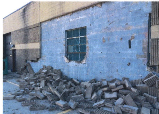
Figure 1 - Wall failure at west façade
