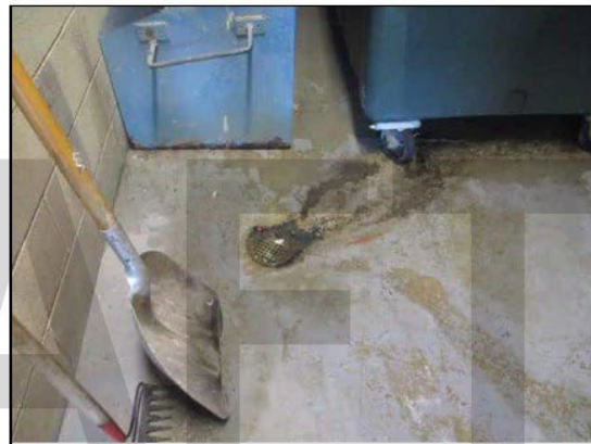
34. Floor drain in the trash room
