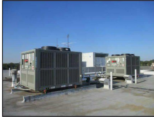
50. Newly installed chillers
