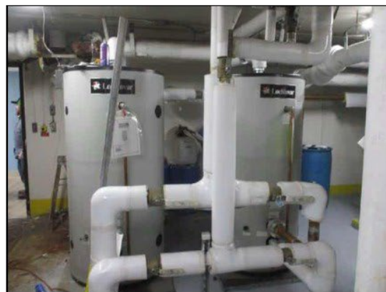
42. Hot water tanks in the boiler room.
