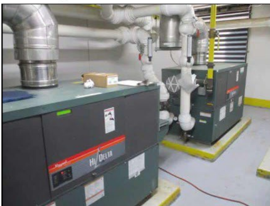
41. Typical boilers in the boiler room.
