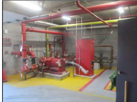
32. Fire suppression equipment.
