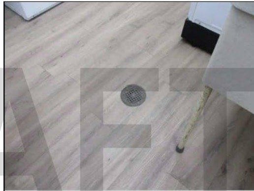
52. Floor drain in the laundry room
