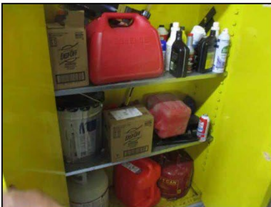
29. Gasoline and oil in a flammable cabinet in the maintenance shop.
