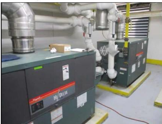
41. Typical boilers in the boiler room.
