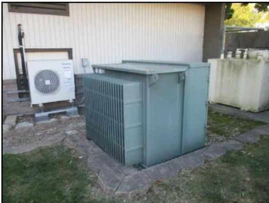
13. Pad-mounted transformer slightly west of the southwestern corner of the Property building.
