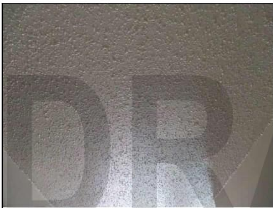
57. Typical spray-applied acoustical ceiling texture (suspect asbestos) in a unit.
