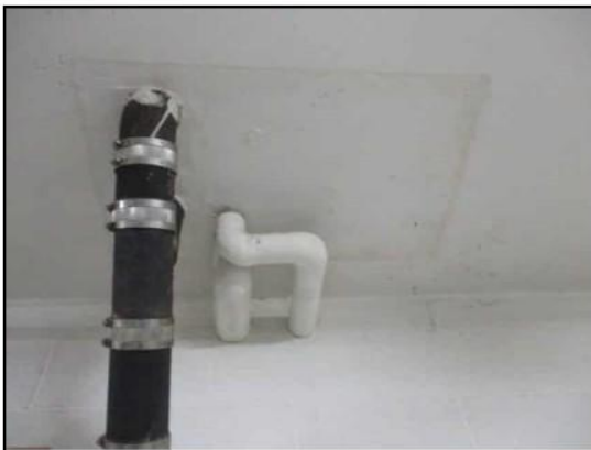
35. Muddled elbows (suspect asbestos) in the maintenance area
