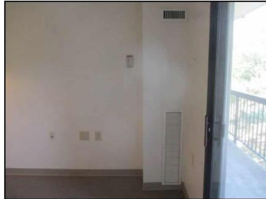
56. Typical fan coil grille and return vent in a unit.
