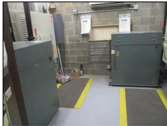
36. Hydraulic elevator service room
