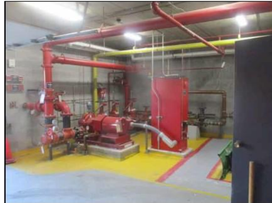
32. Fire suppression equipment.
