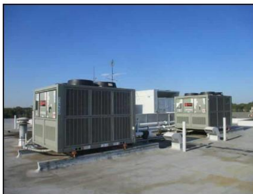
50. Newly installed chillers
