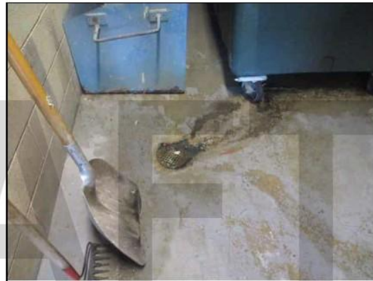
34. Floor drain in the trash room
