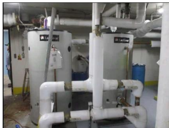
42. Hot water tanks in the boiler room.
